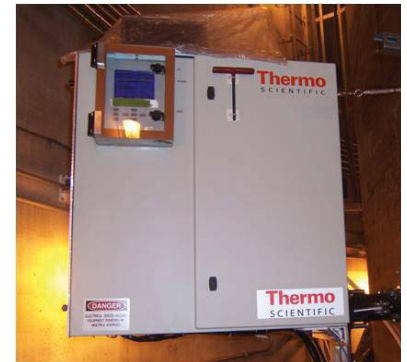
Figure 4: View of the alpha test installation at a coal-fired power plant.
